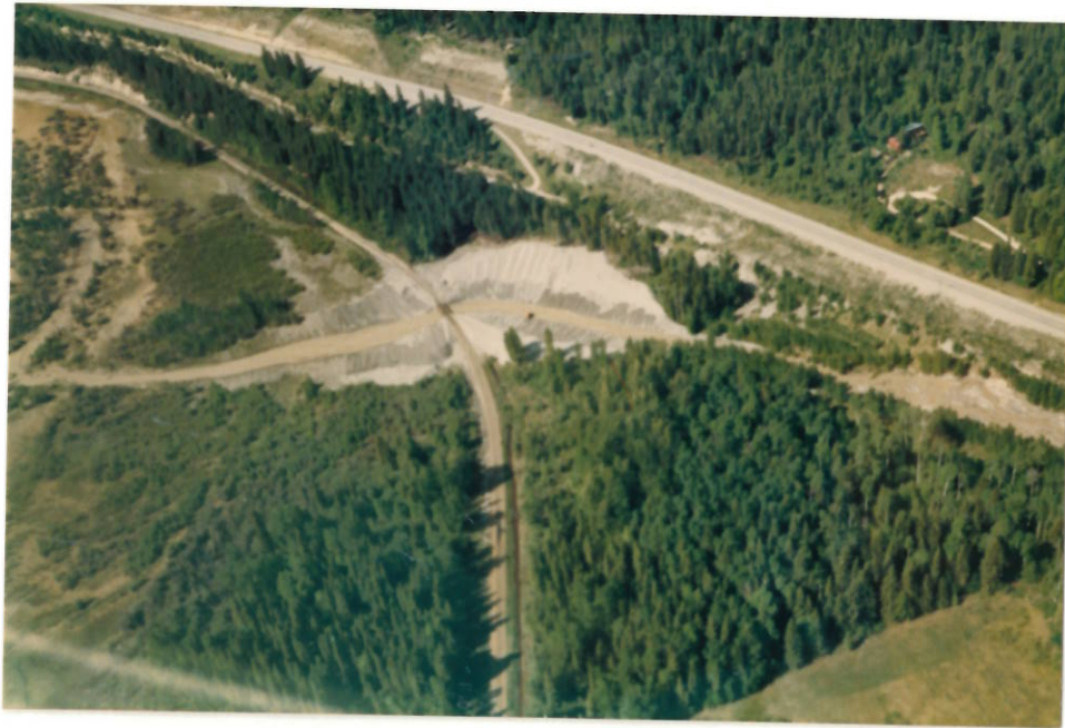
Photo #7 - Bulldozer working to prevent washout of CPR Bridge
